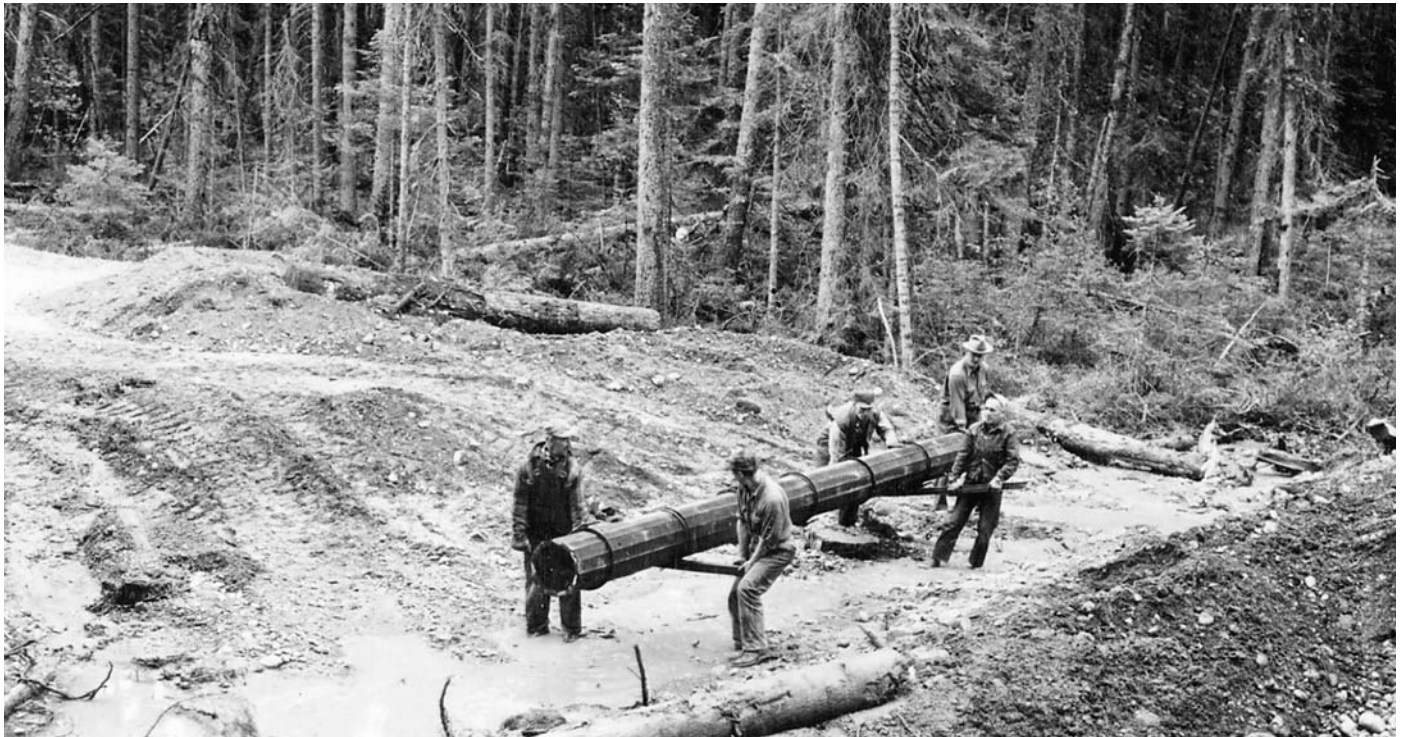
A road construction crew working on Willow River Road east of Prince George opens up central Interior forests for development in 1956.
